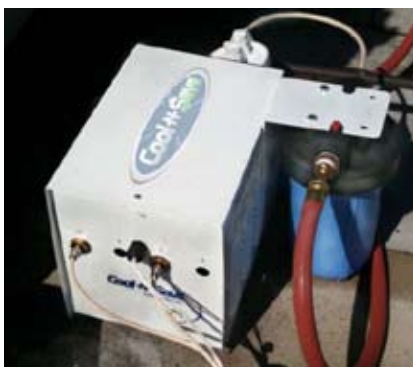
Top: A typical Greenway pre-cool commercial installation with the micro nozzle array.
